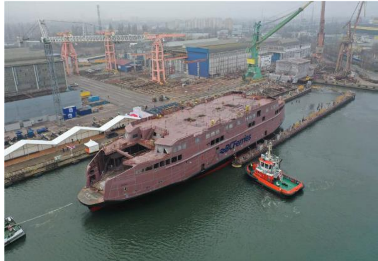
Construction of the Salish-Class vessels (2016), at Remontowa Shipbuilding S.A. in Gdansk Poland.
