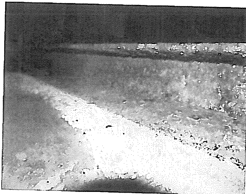
18. DBT 4 corroded bottom longitudinal
