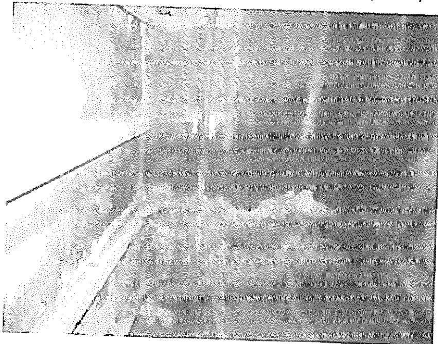
22. Side ballast tank 2P with signs of corrosion at lower part of bulkheads, sides and bottom structure.
