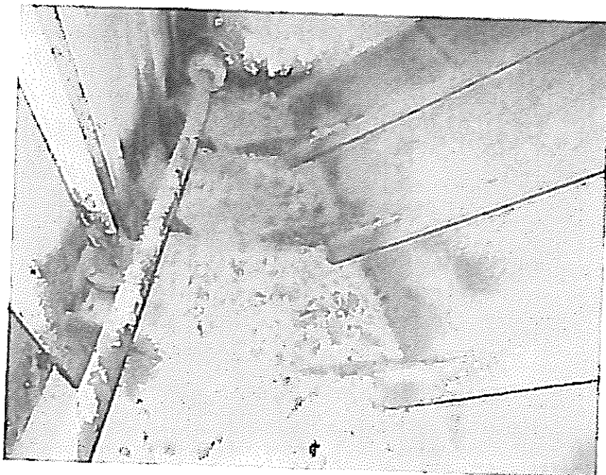
31. Void space no. 1 corroded floor and lower part of bulkheads, side and frames
