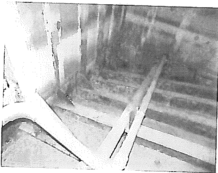
30. Aft peak port side in generally rusty and/or locally corroded condition
