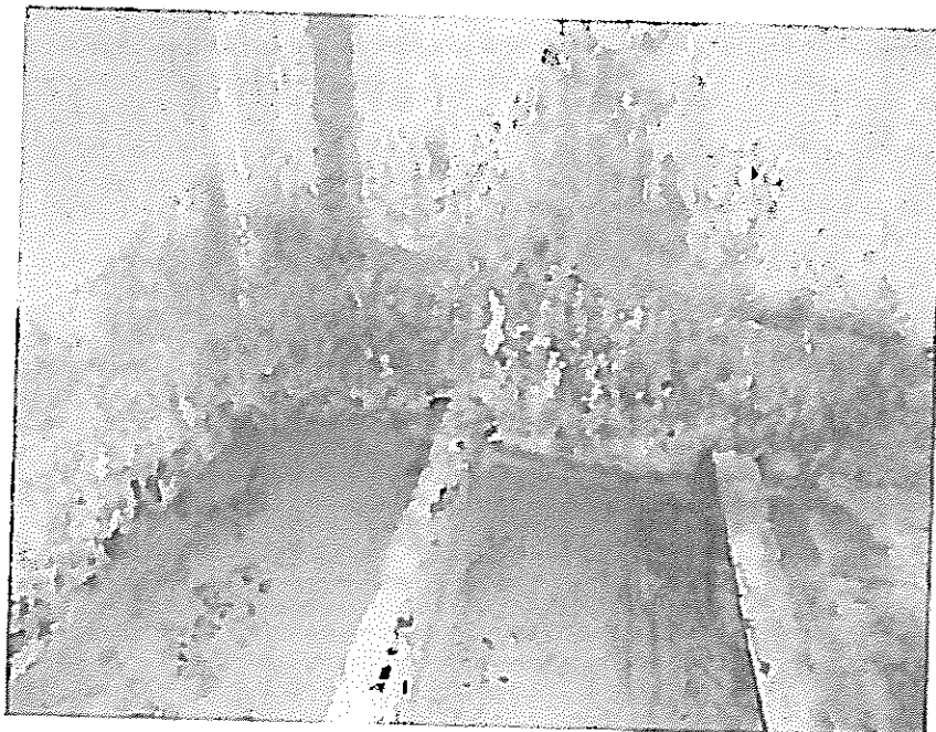
17. DBT 4 corroded steel surfaces
