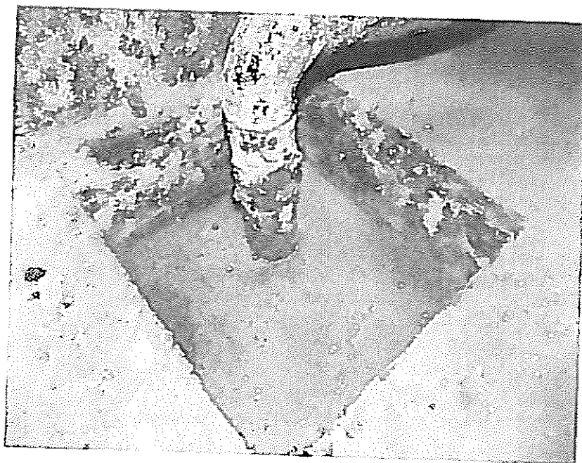
32. Void space no. 1 heavily corroded bilge well and piping
