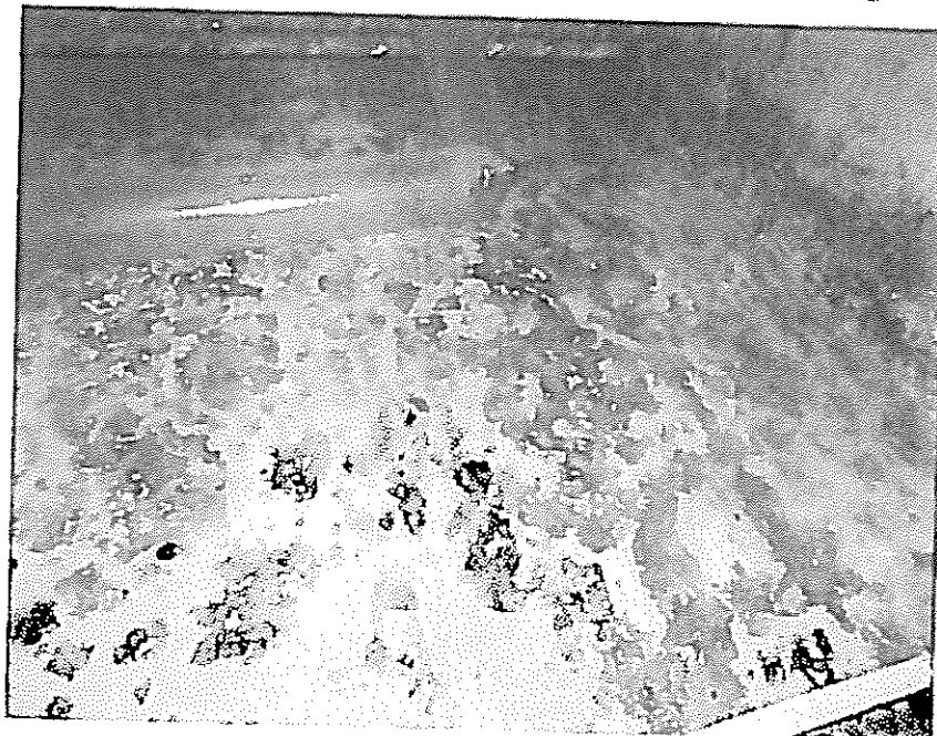
34. Void no. 3 corroded bottom plating
